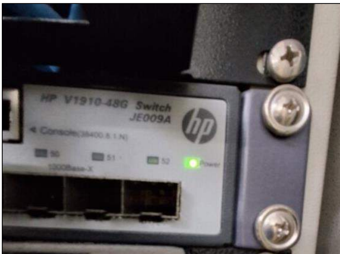
ITEM 030- RACK COM SWITCH
