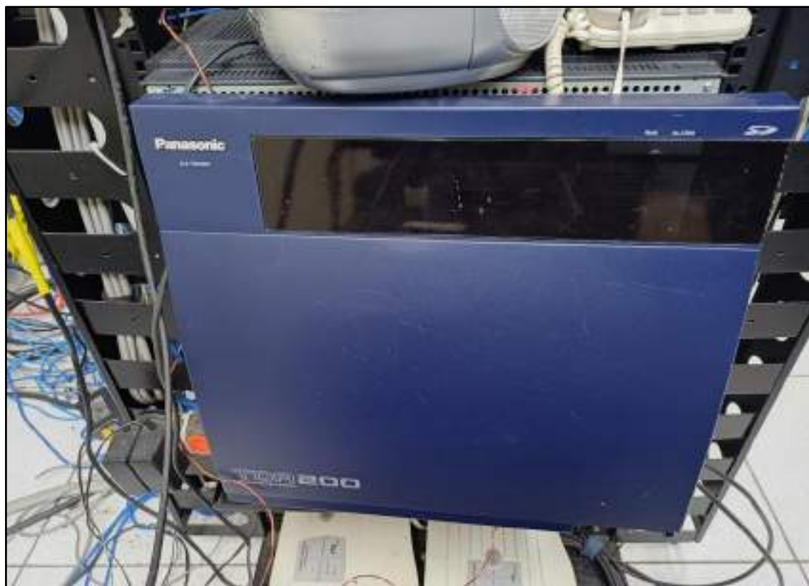
ITEM 089 - PABX PANASONIC TDA200 E RACK
