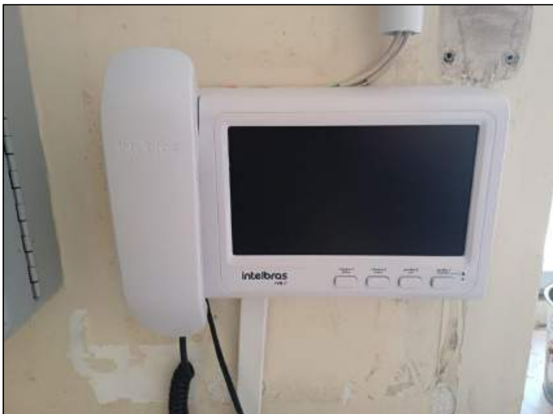
ITEM 165 - INTERFONE INTELBRAS
