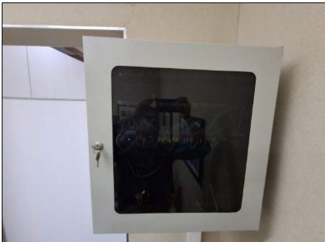
ITEM 030- RACK COM SWITCH
