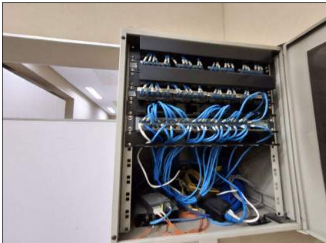
ITEM 030- RACK COM SWITCH
